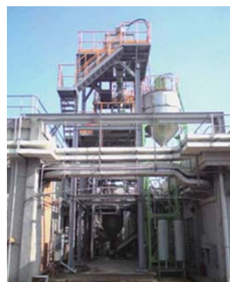
▲ The Acid Hydrolysis Pretreatment Facilities of Ton-Scale Pilot Plant in INER
