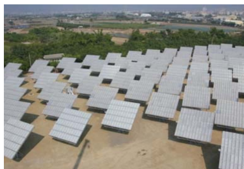
▲ The MW-Grade On-grid Type HCPV Demonstration Plant
