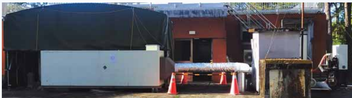
Air conditioning system of adsorption rotary wheel
